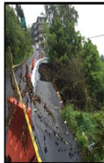
FIGURE 1C. LANDSLIDE LOCATION IN YEH MAMPAH VILLAGE SUB DISTRICT OF KINTAMANI
