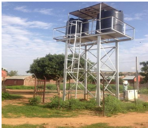
PLATE 3A. OVERHEAD TANK
